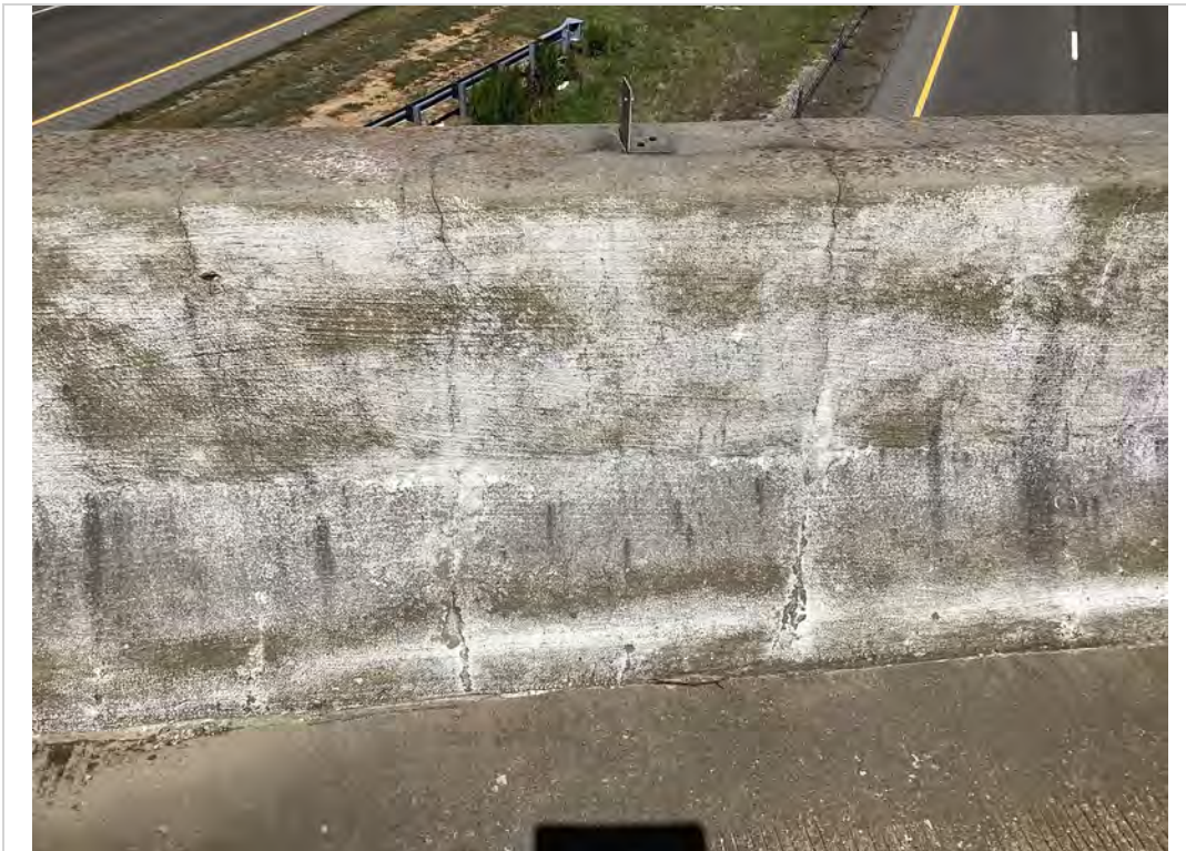
Span 2 parapet cracks
