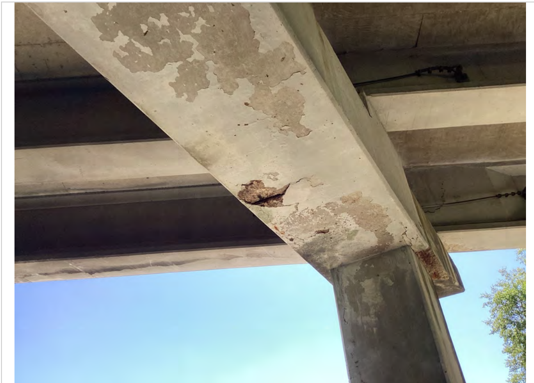
Bent # 3 cap, spall to steel area(s)
