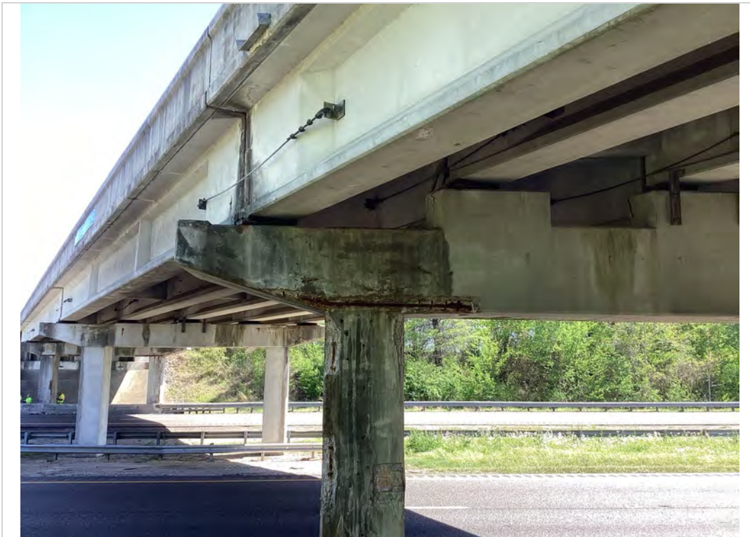
Bent # 3 poor bearing under A-E
