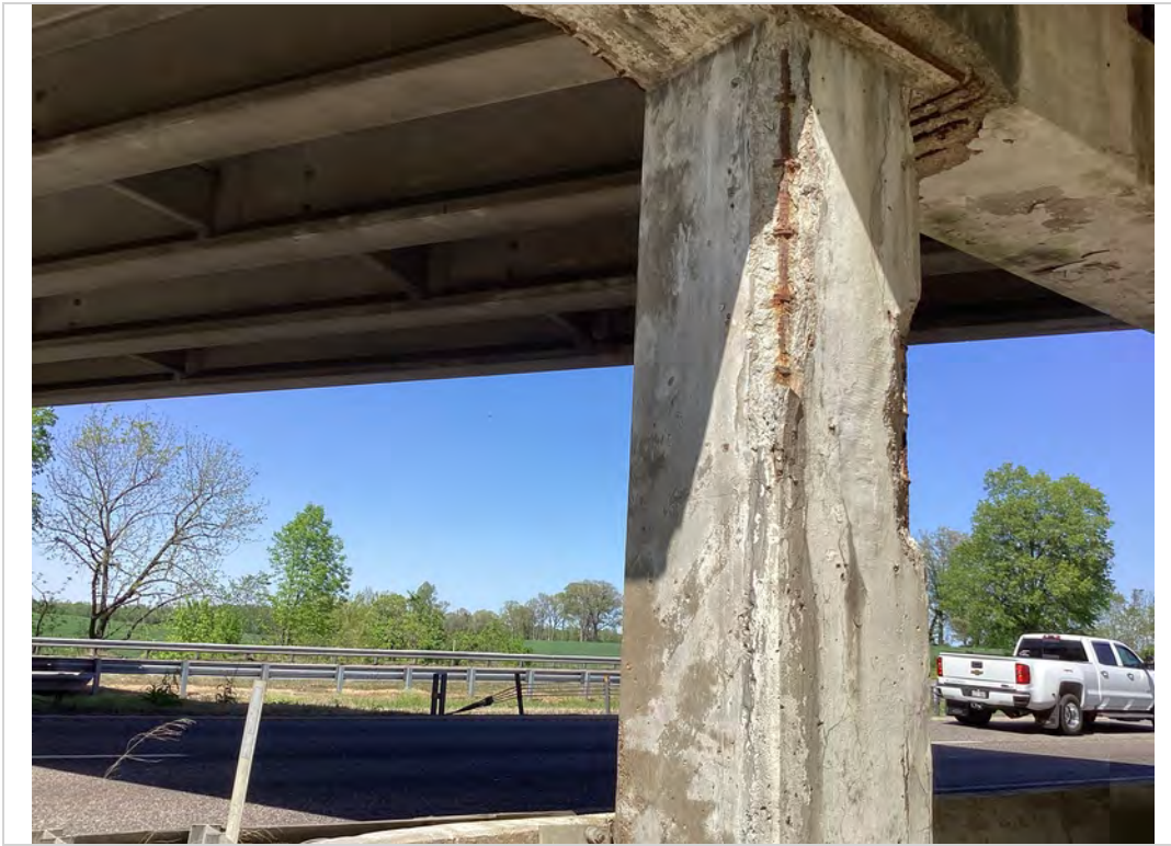
Bent 1 Column A spalled to steel on Left side
