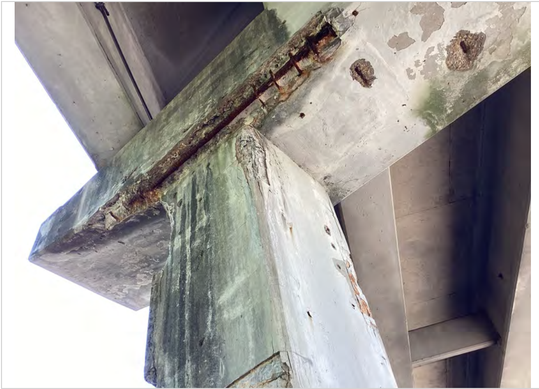
Bent # 3 cap, spall to steel area(s)
