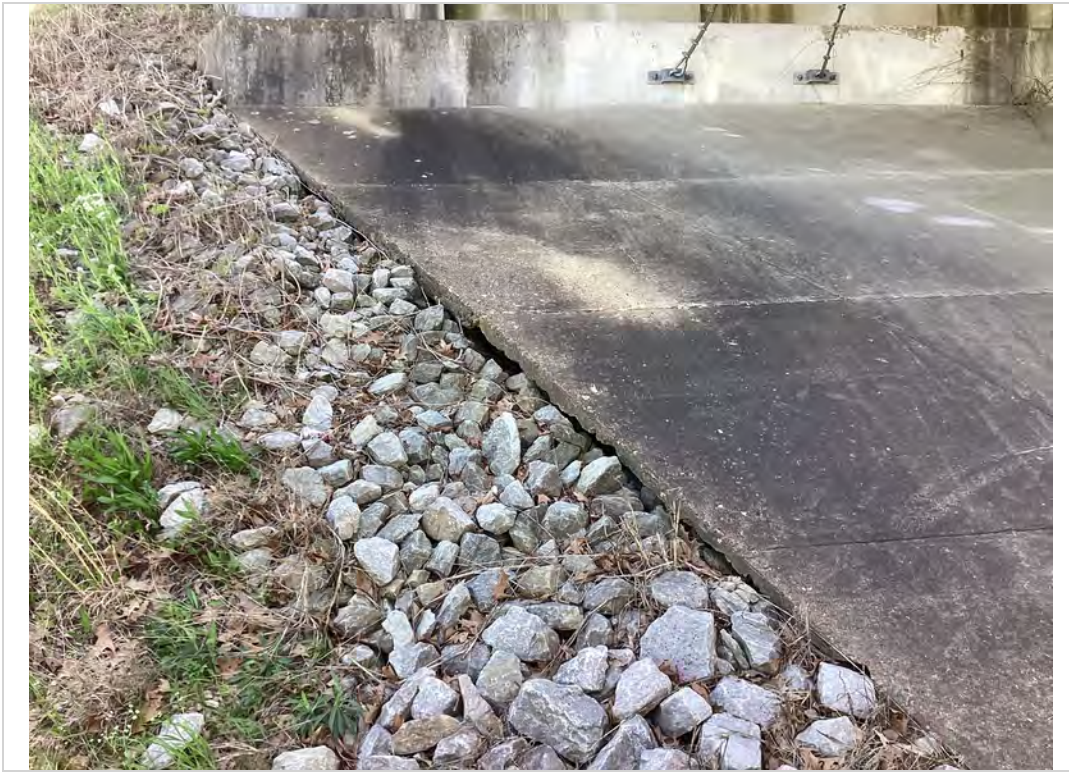
Abutment 1 embankment washing at right side slope paving
