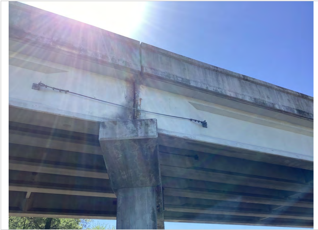
Span 2 concrete I-beam "E" spall to steel
