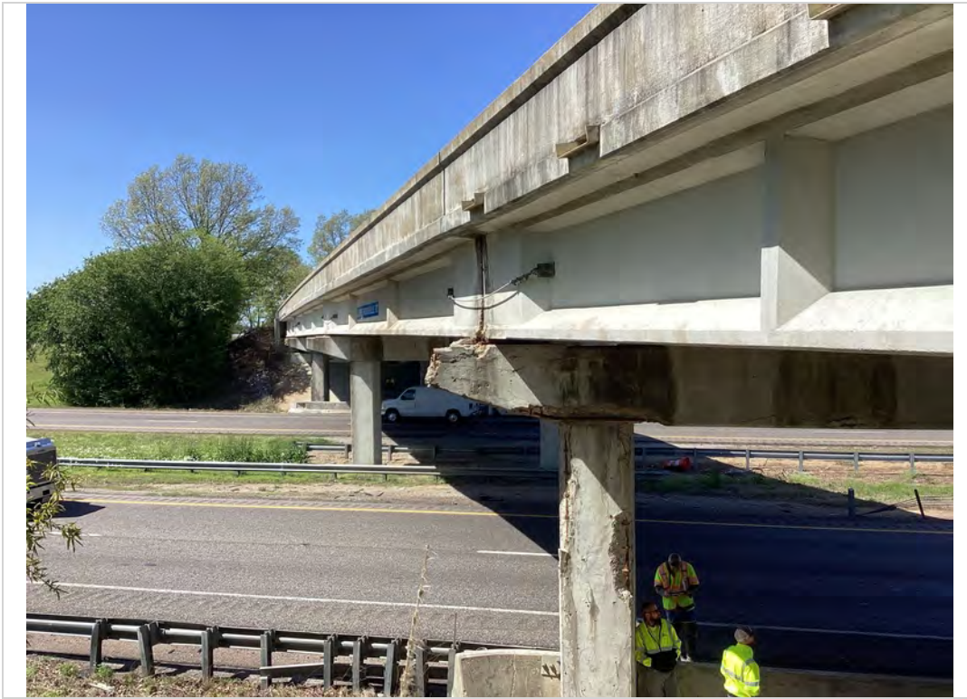
Span 2 concrete I-beam "A" spalling
