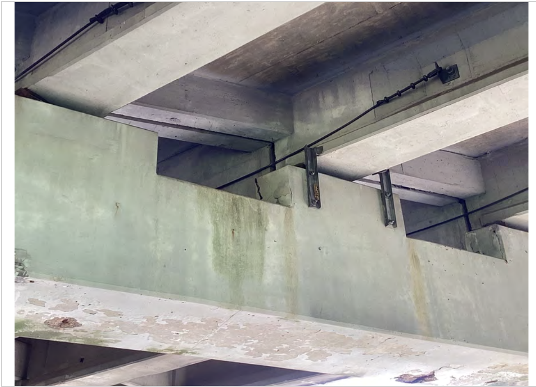
Bent # 3 cap, impending spall area(s)
