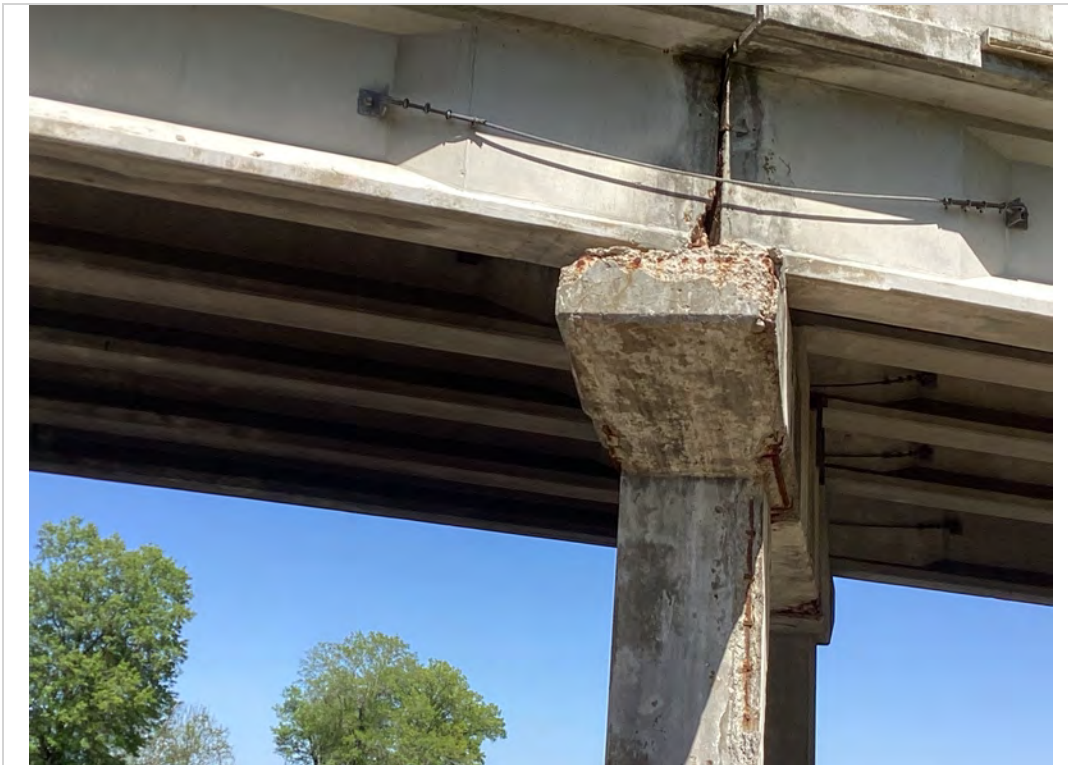
Bent 1 Left end of of Cap spalled
