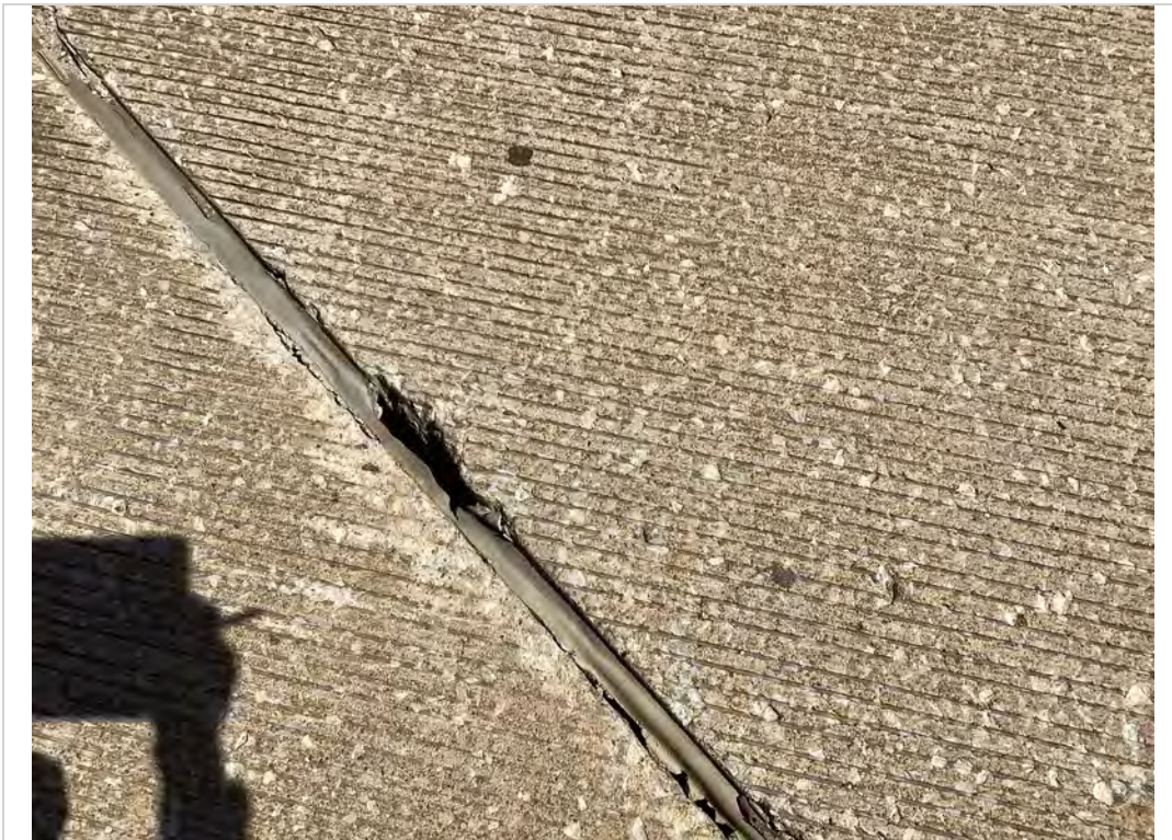
Span 3 joint and spall
