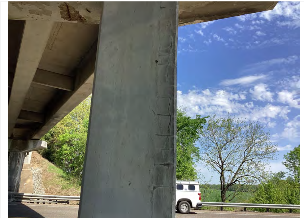
Bent 2 column b cracking
