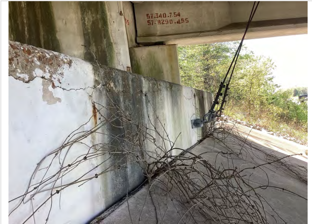
Abutment 1 fine cracks up to 1/16"
