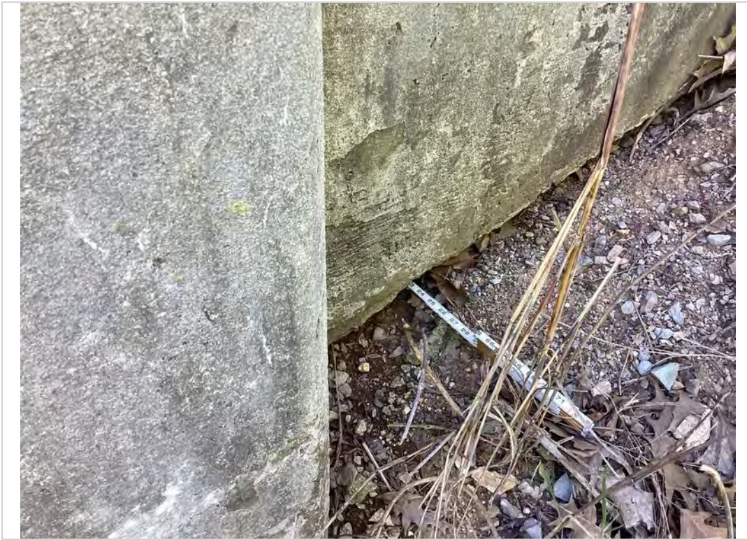
Abutment # 2, wing wall , Right side , Embankment washing below and back under wing
