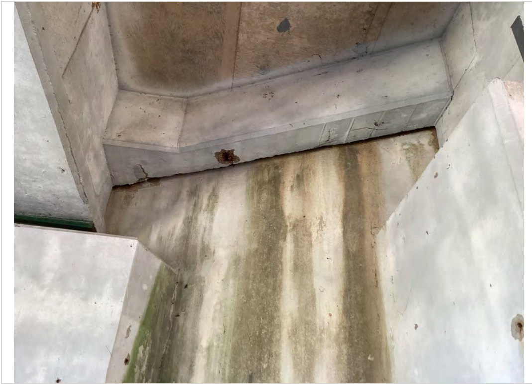
Span 1 bottom deck looking back diaphragm impending spall and spall to steel
