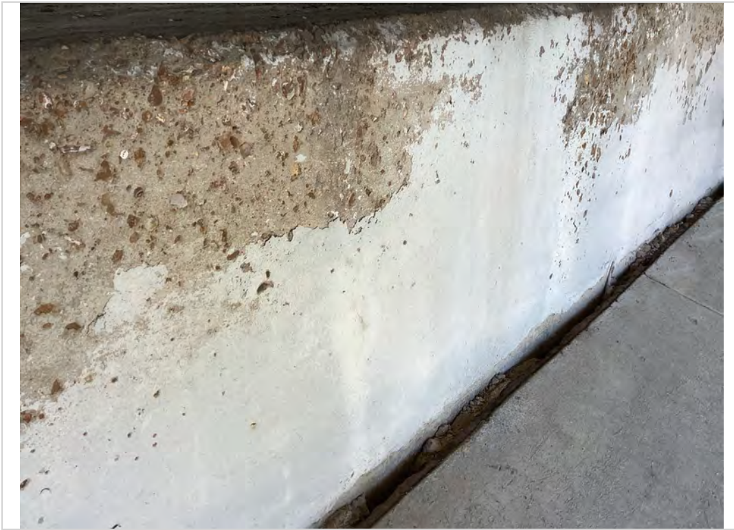
Abutment # 2 cap, scaling
