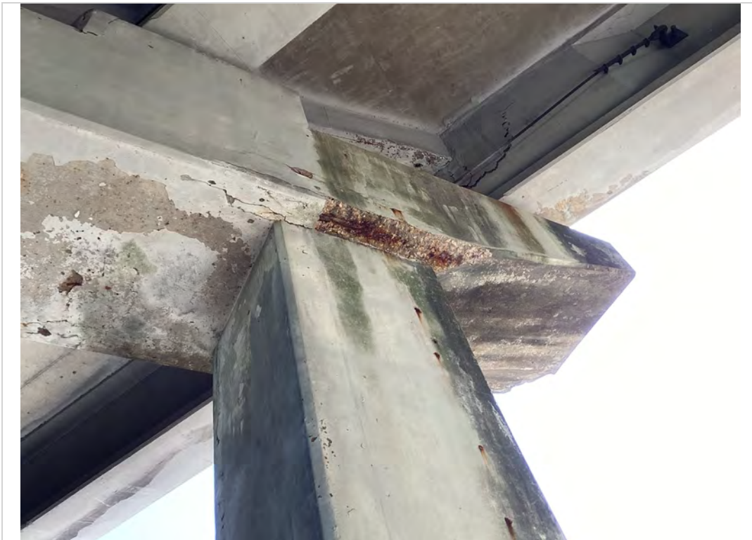
Bent # 3 cap, spall to steel area(s)
