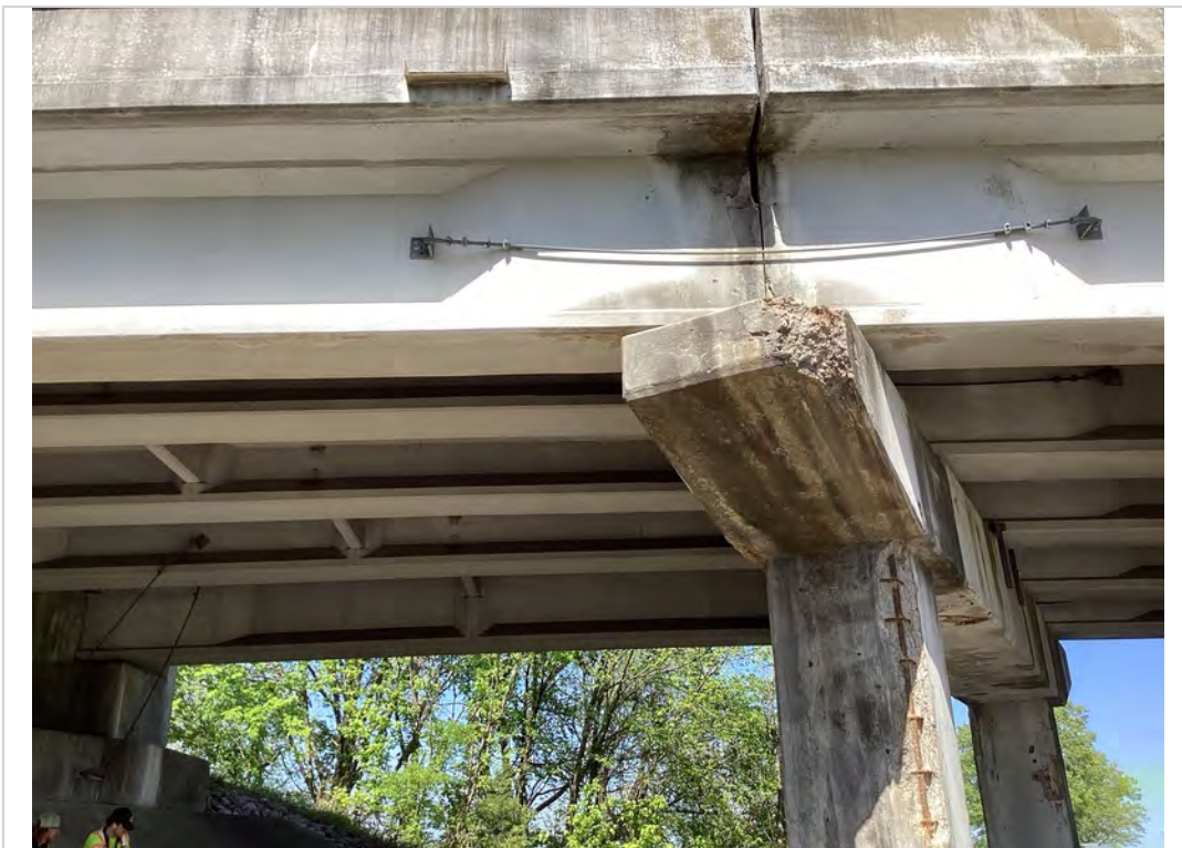
Bent 3 cap spalled to steel on Left end
