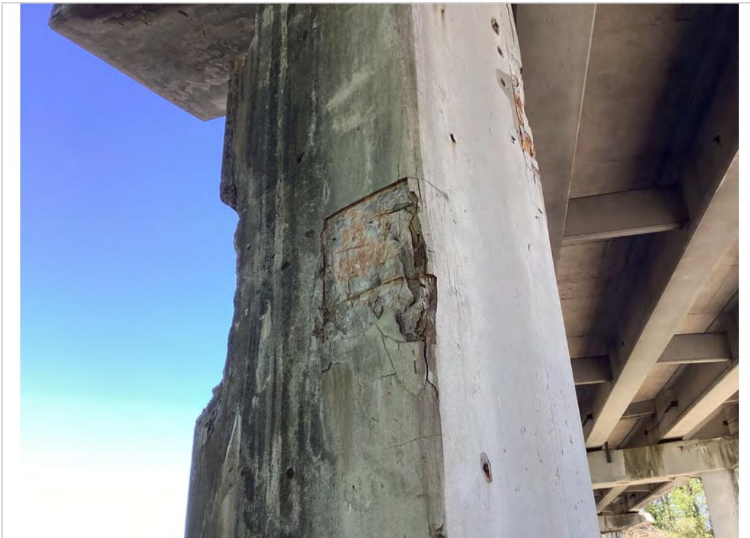
Bent # 3 cap, spalling area(s) in patched area
