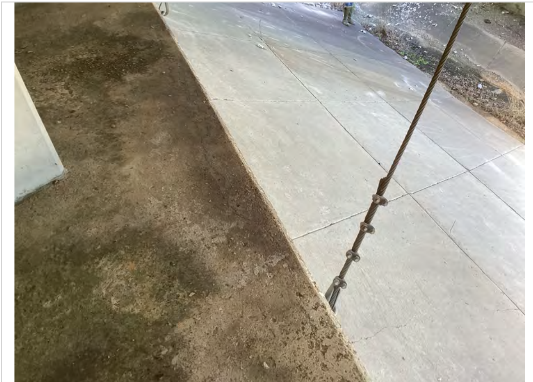
Abutment # 2 cap, fine crack(s)
