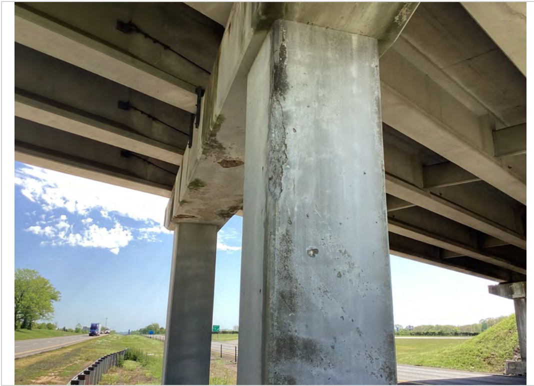
Bent 2 column a spall
