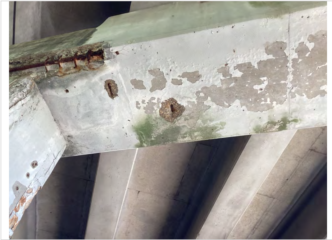
Bent # 3 cap, spall to steel area(s)
