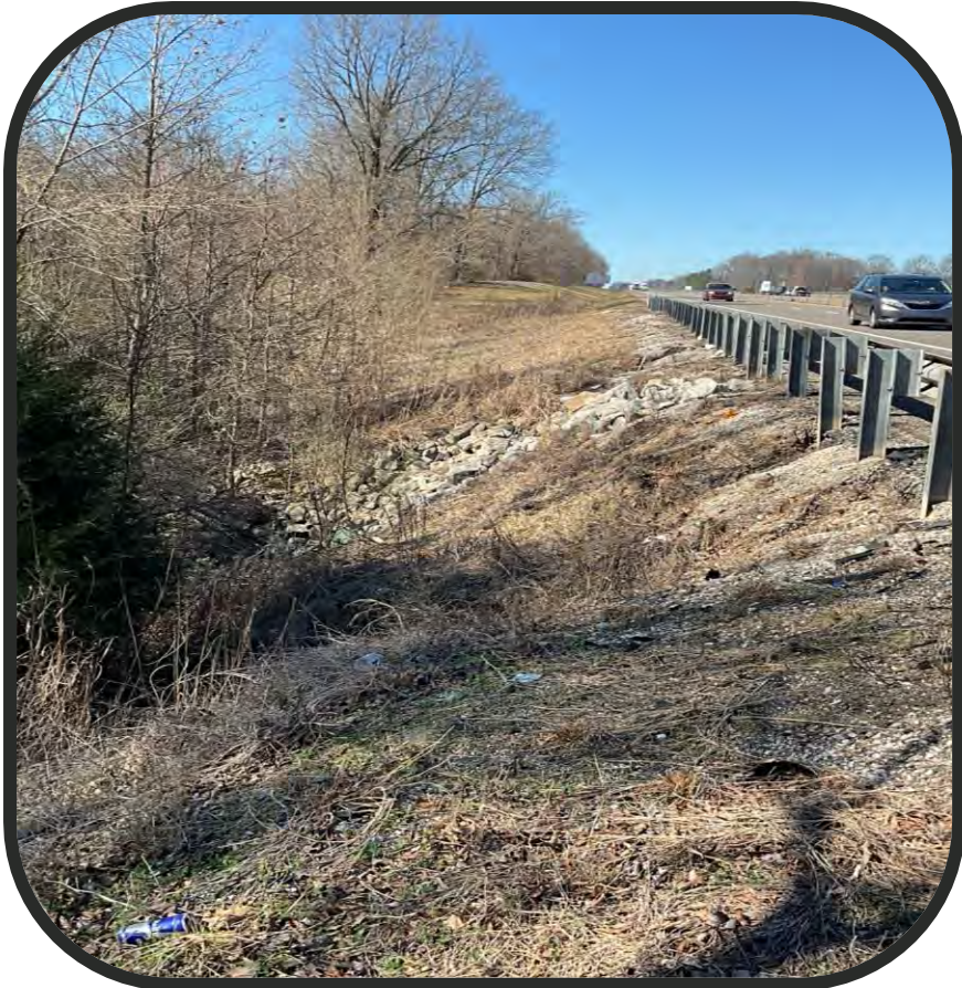
Embankment Erosion Along I-40 EB
