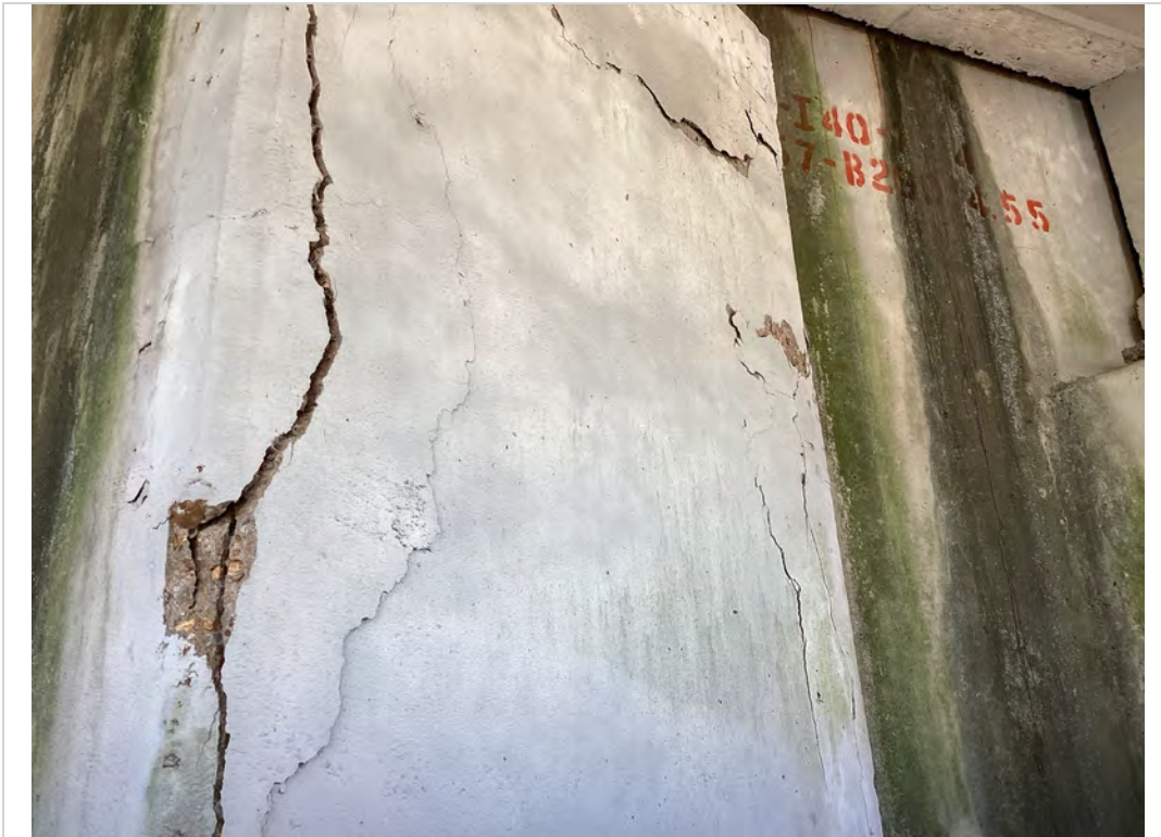
Abutment 1 riser block impending spalls
