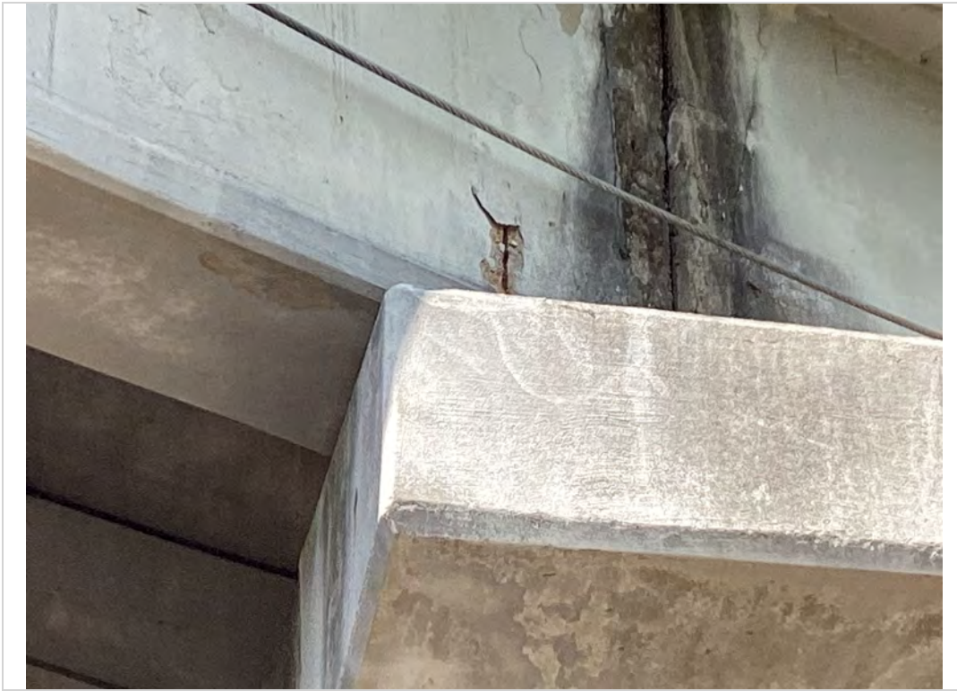
Span 3 beam e spall to steel
