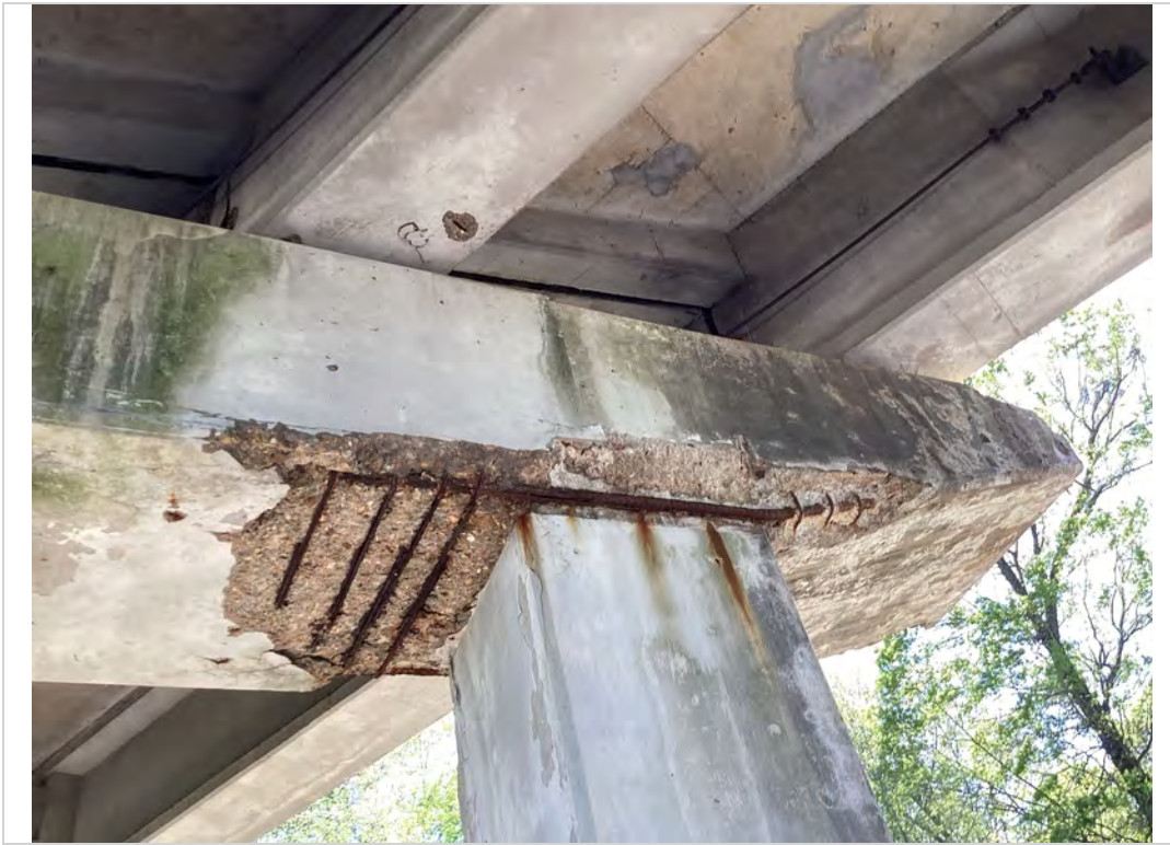
Bent 1 cap spalled to steel on rear side over pile A
