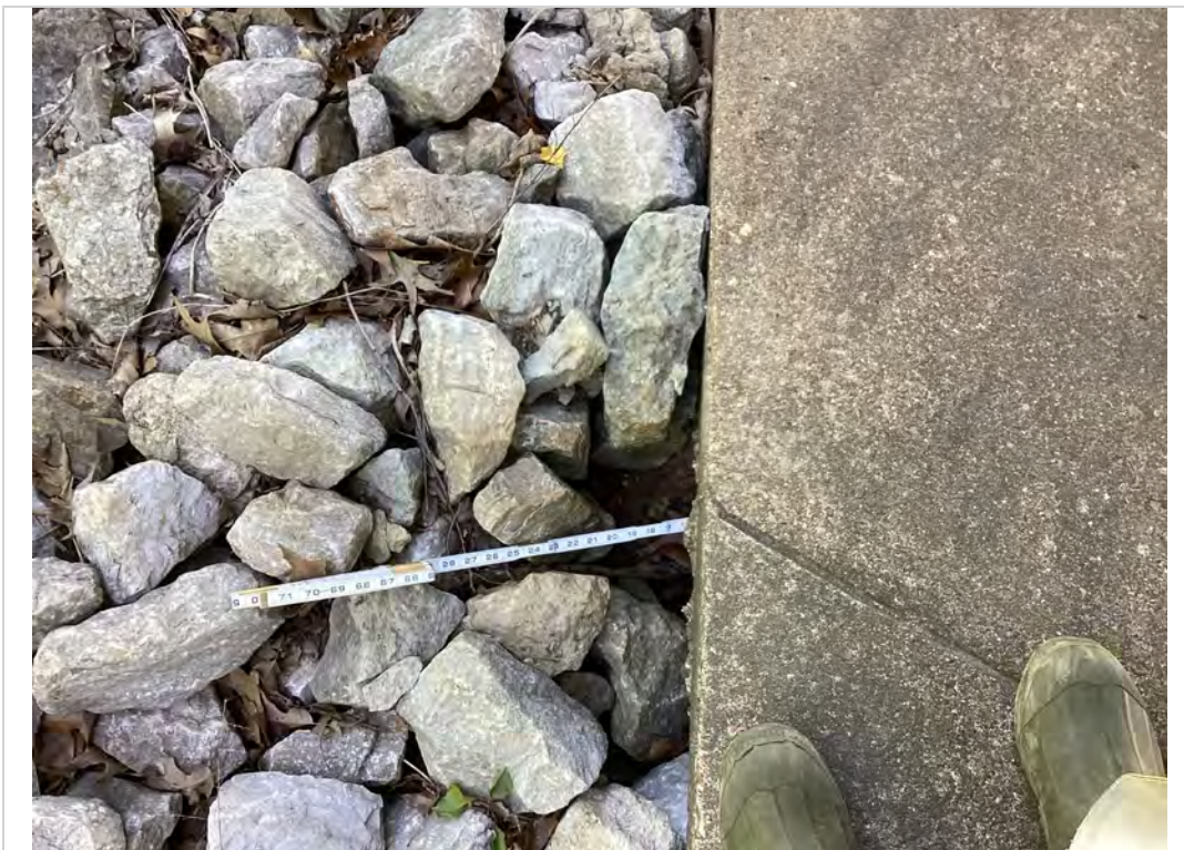
Abutment # 2 embankment washing, Embankment washing below and back under slope pavement
