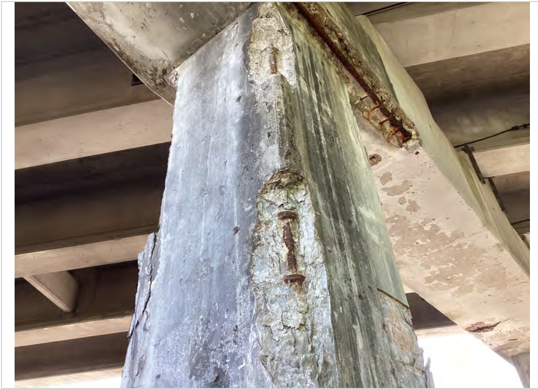
Bent # 3 Column(s) B, spall to steel area(s)
