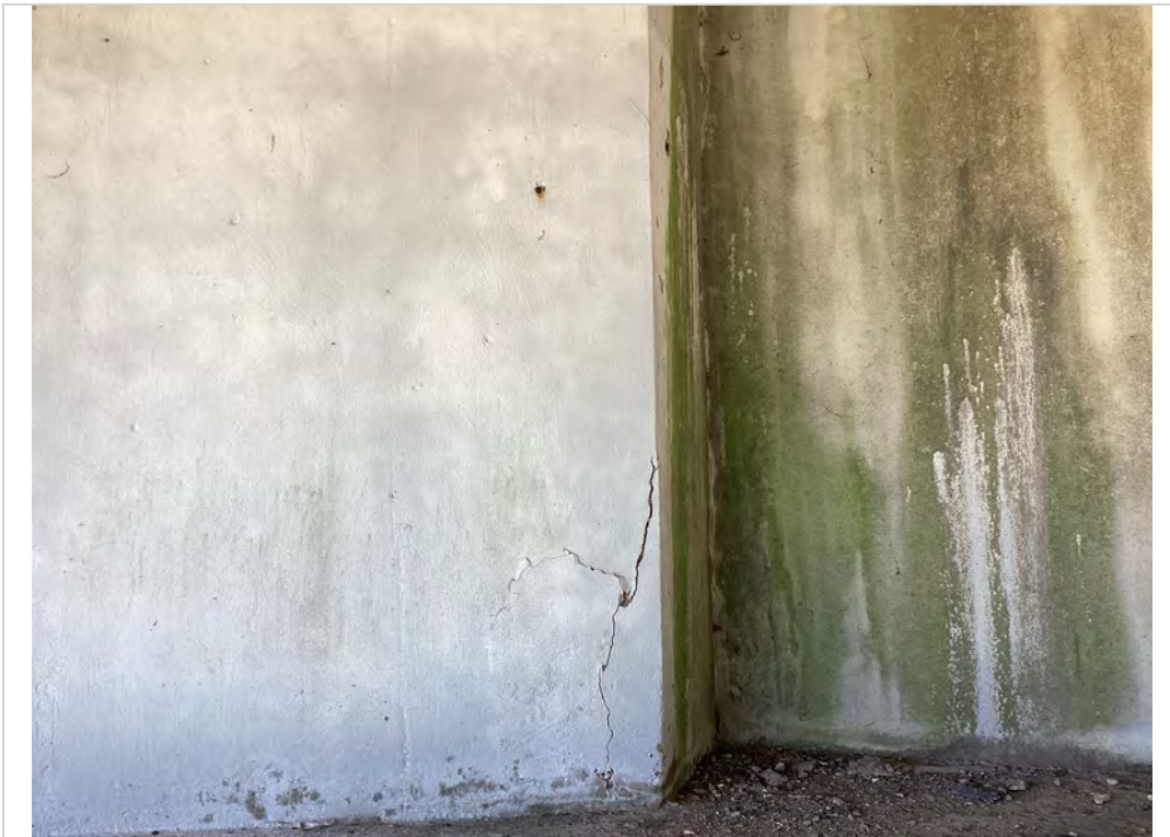
Abutment 1 riser block fine crack up to 1/16"
