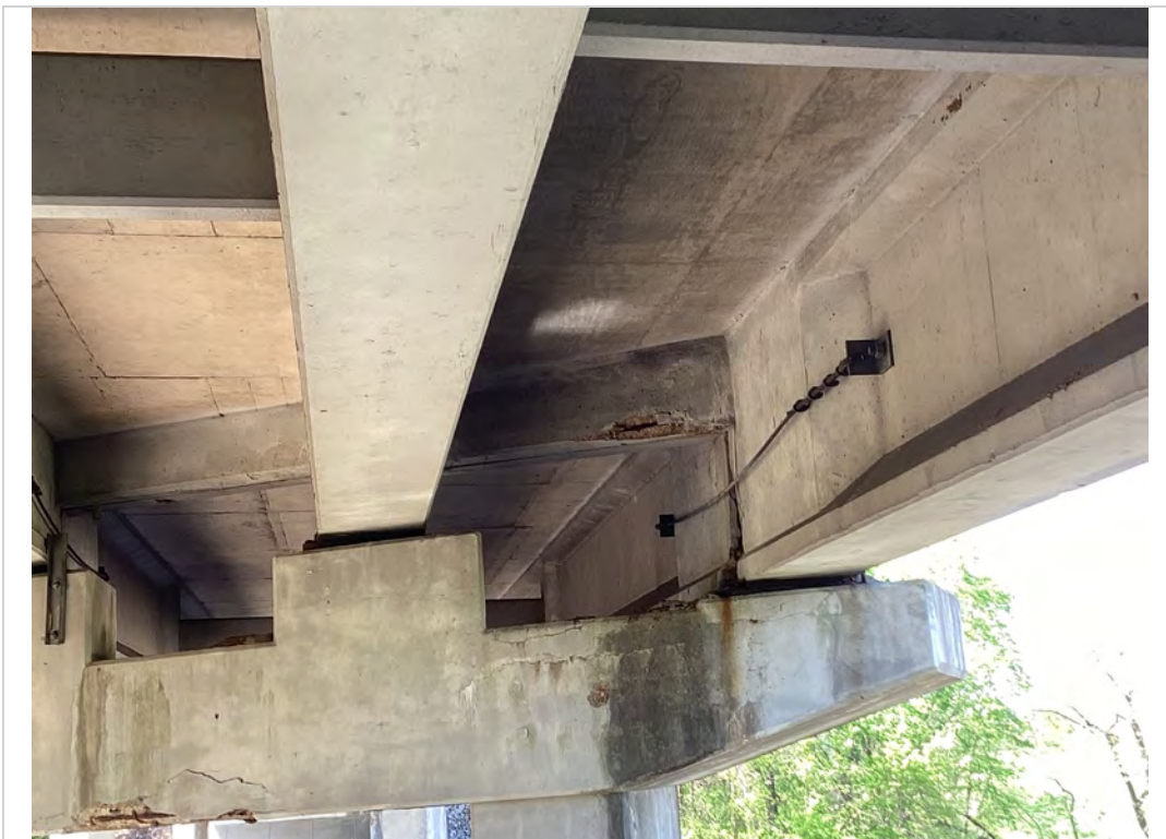
Span 1 bottom deck looking ahead diaphragm spall to steel
