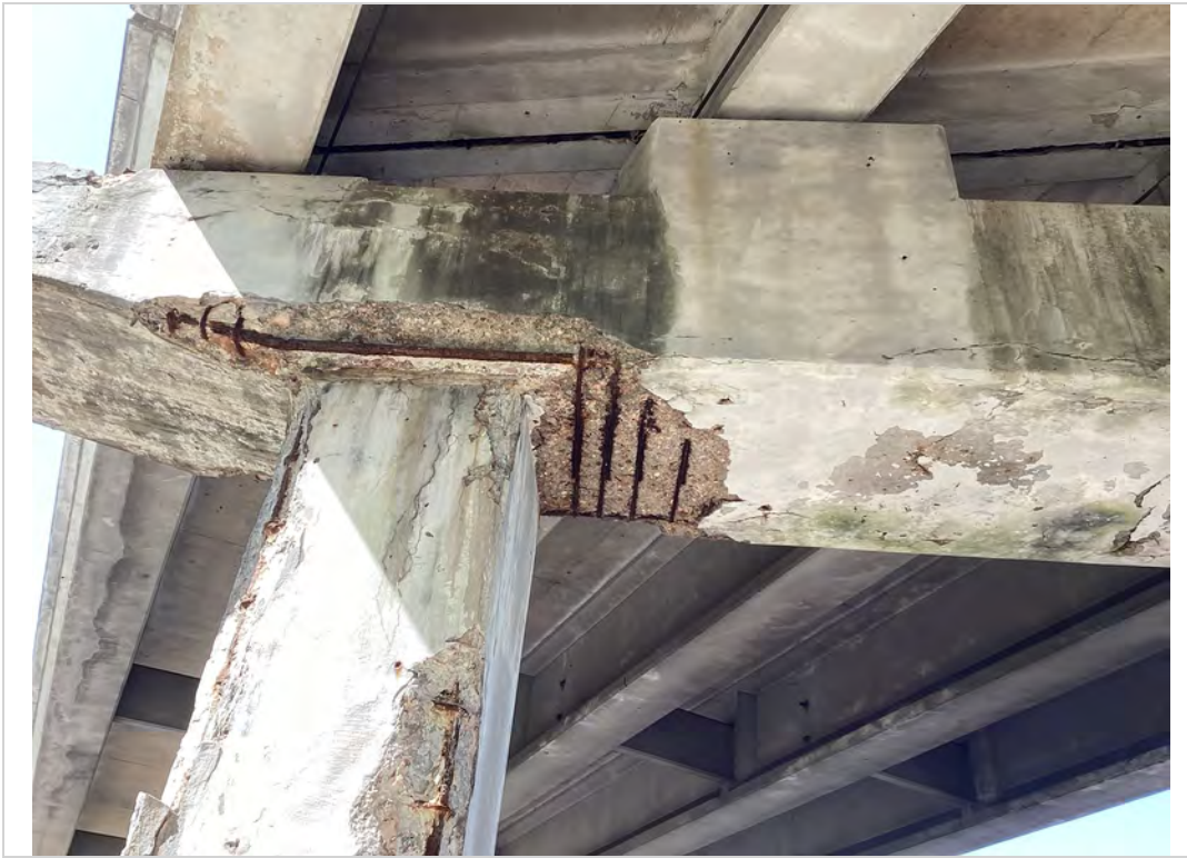
Bent 1 Cap spalled to steel on Left side and on the bottom
