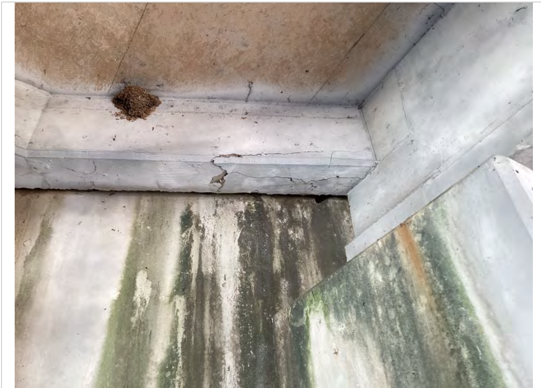
Span 1 bottom deck looking back diaphragm impending spall
