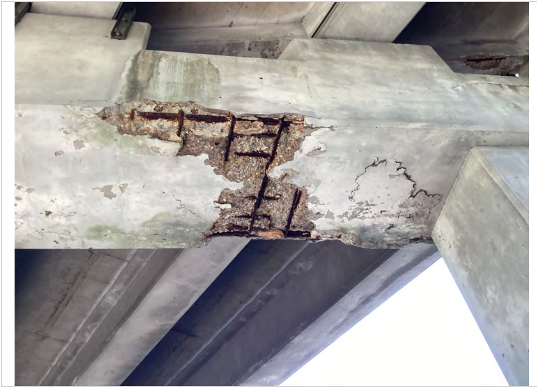
Bottom of cap Bent 1 spalled to steel and beginning to Spall
