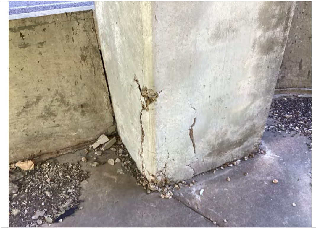
Bent 1 column B beginning to Spall. Front side
