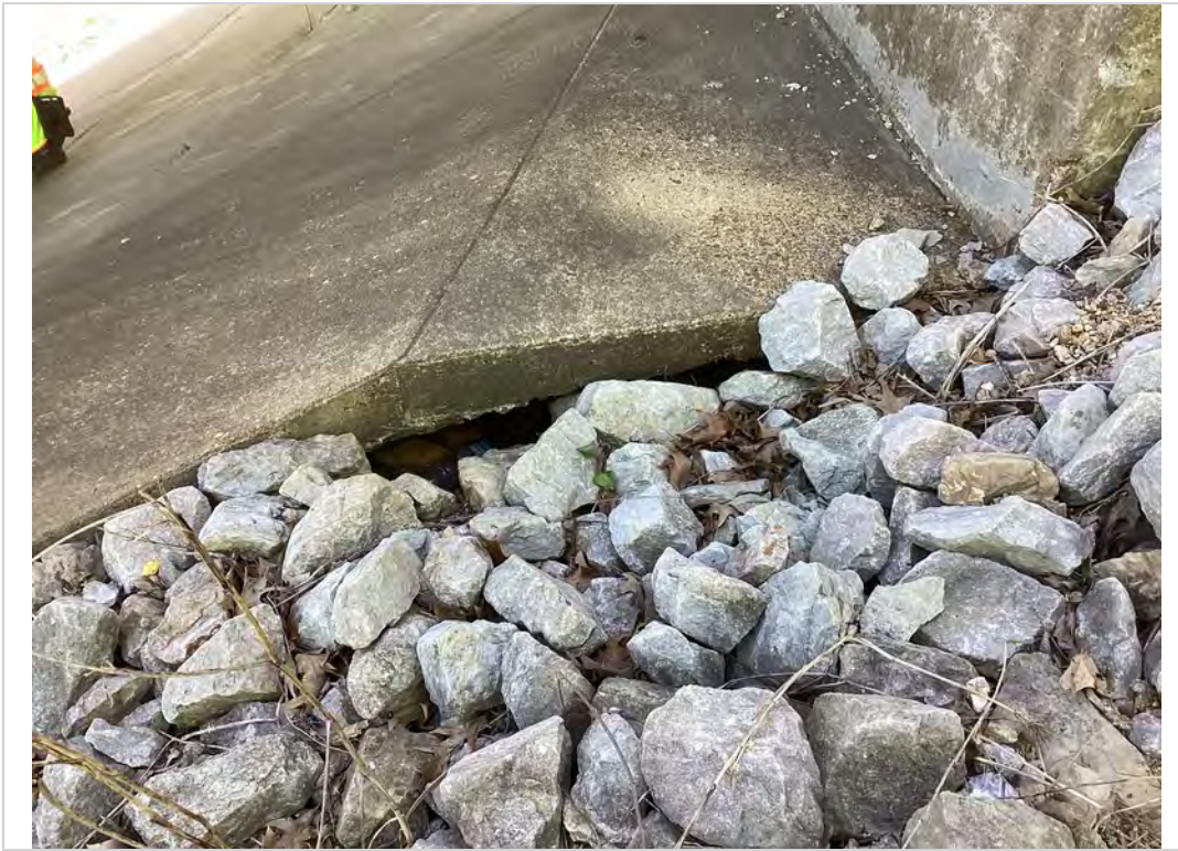
Abutment # 2 , Embankment washing below and back under slope pavement
