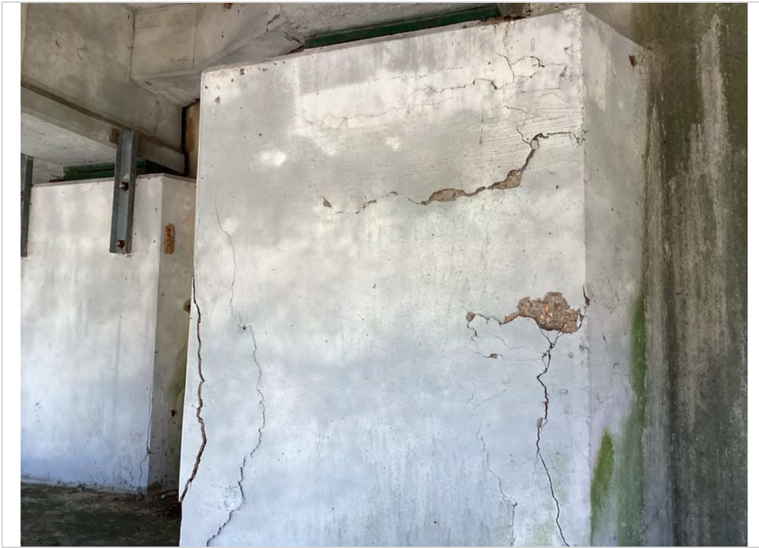
Riser block on abutment 1 impending spall and 1/8" cracking
