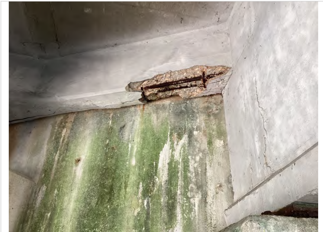
Spall steel on back wall span 4
