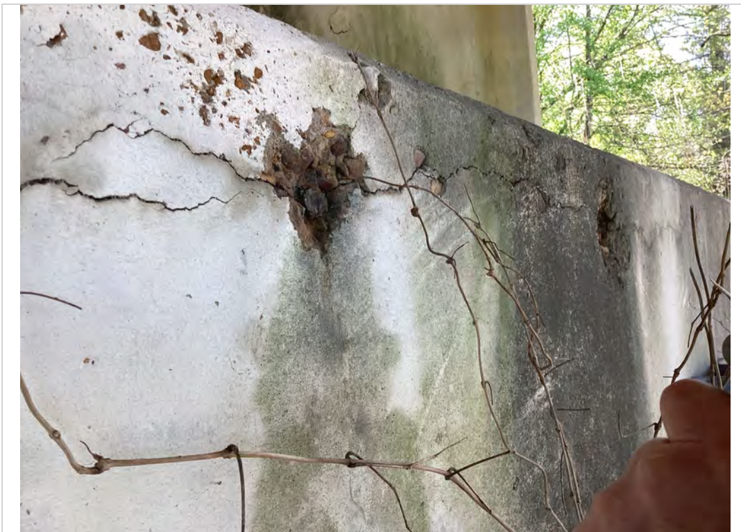
Abutment 1 cap Spall to steel
