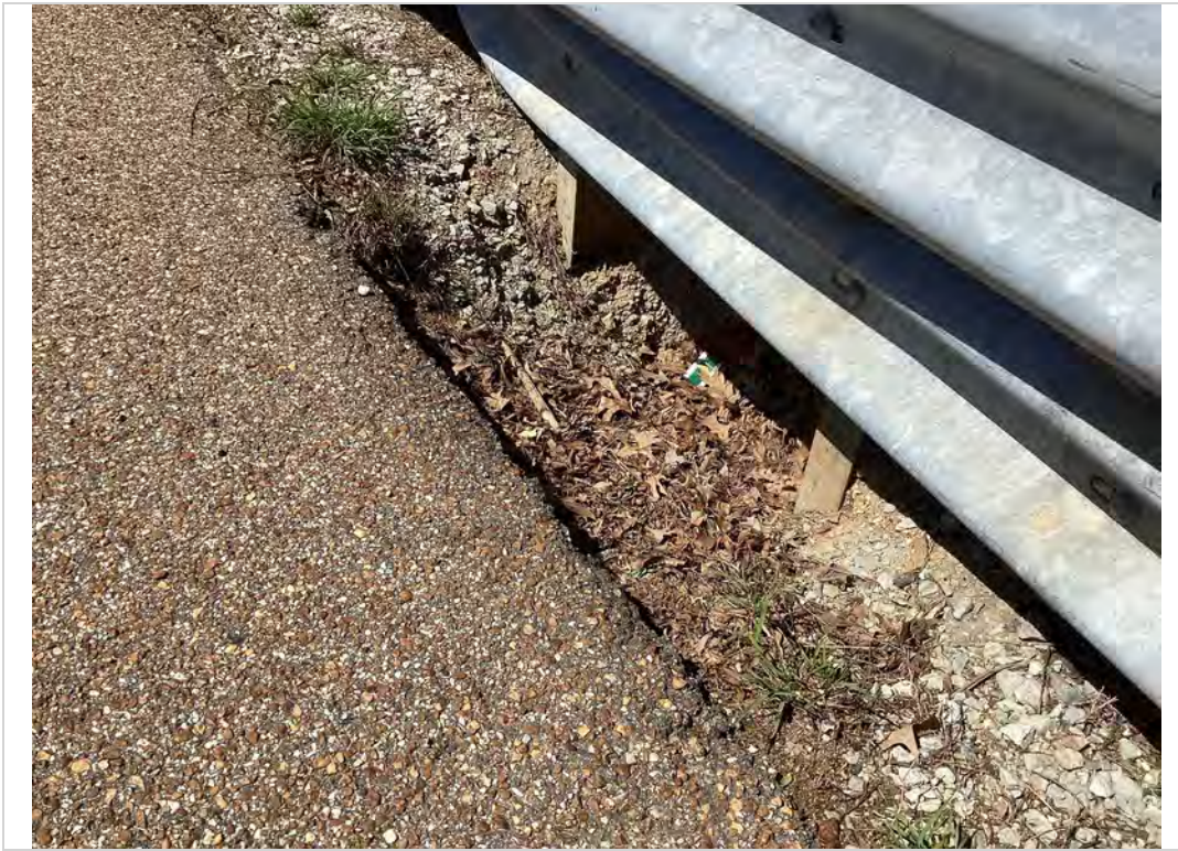
Approach 2 right embankment washing
