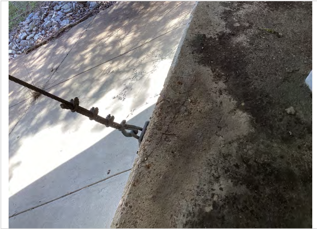
Abutment # 2 cap, fine crack(s)
