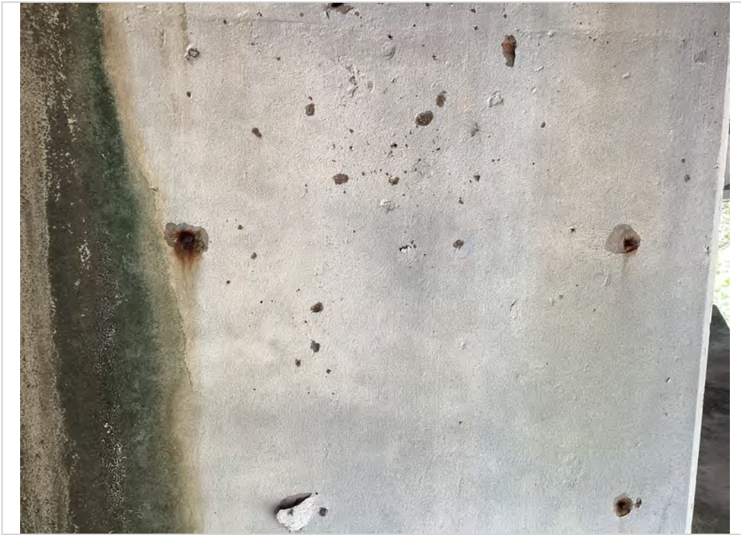
Abutment # 2 pop outs, surface spall
