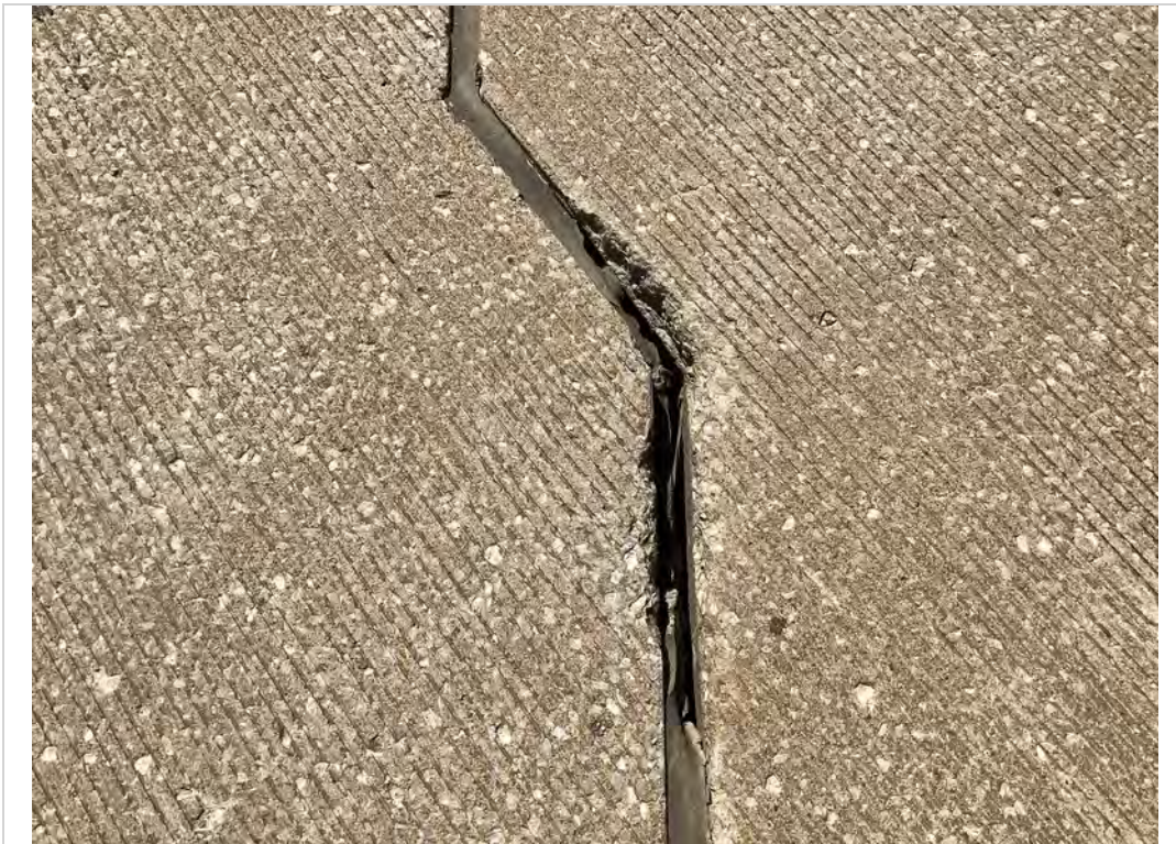
Span 1 joint material missing
