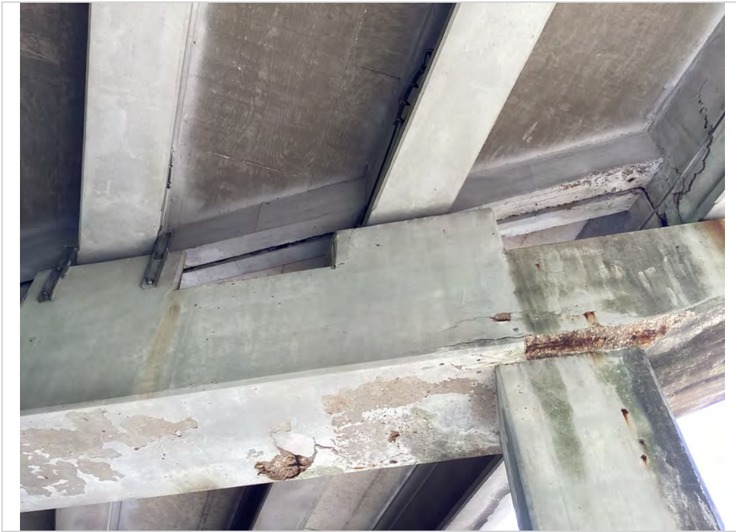
Bent # 3 cap, spall to steel area(s) , spalling area(s) , fine crack(s)
