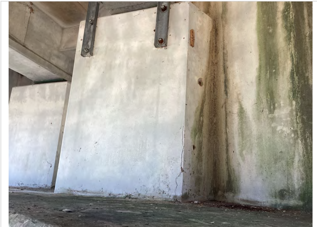
Abutment 1 riser block fine crack up to 1/16"
