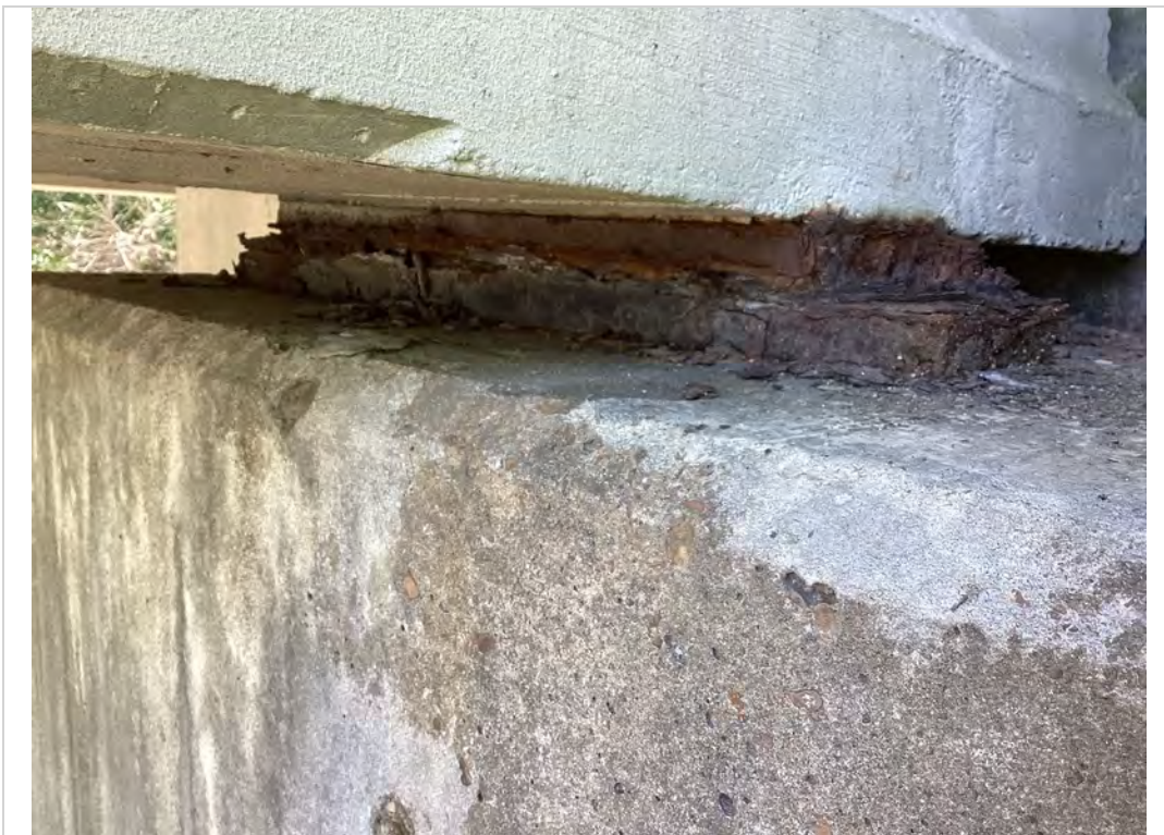
Abutment # 2 poor bearing under beam E
