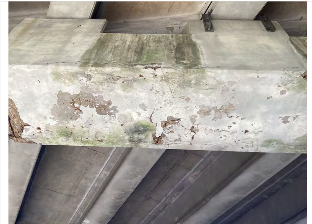
Bottom of cap Bent 1. Delamination
