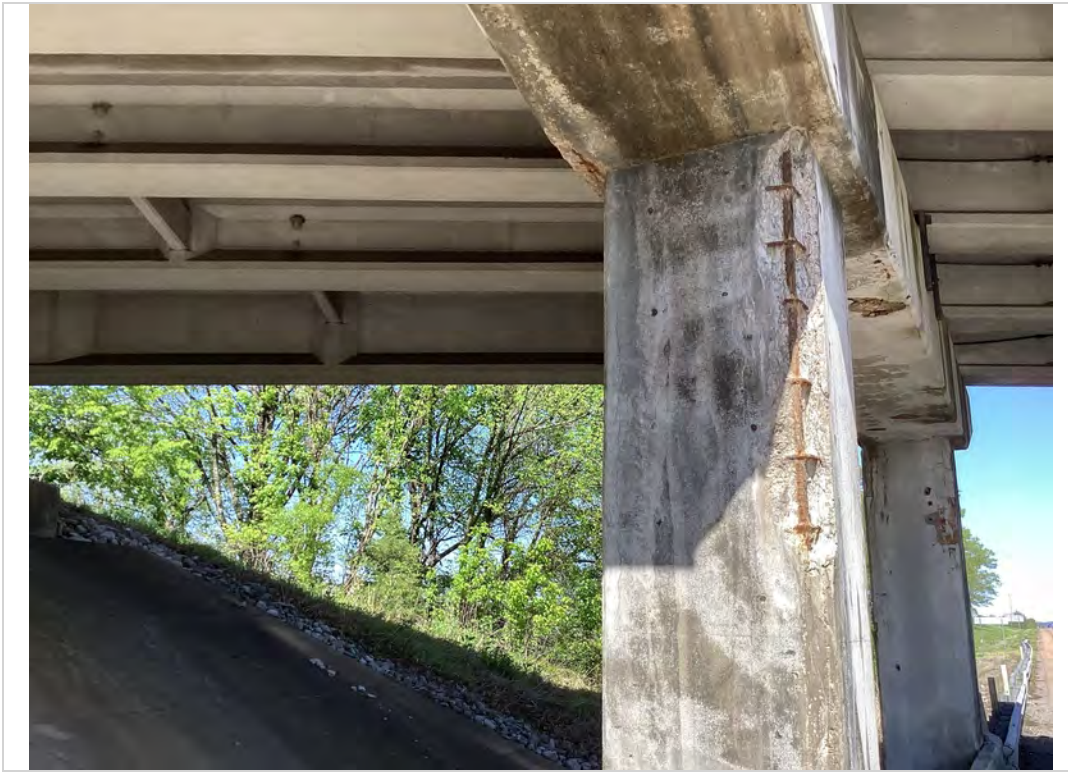
Bent 3 column A spalled to steel on Left side Direction of Route
