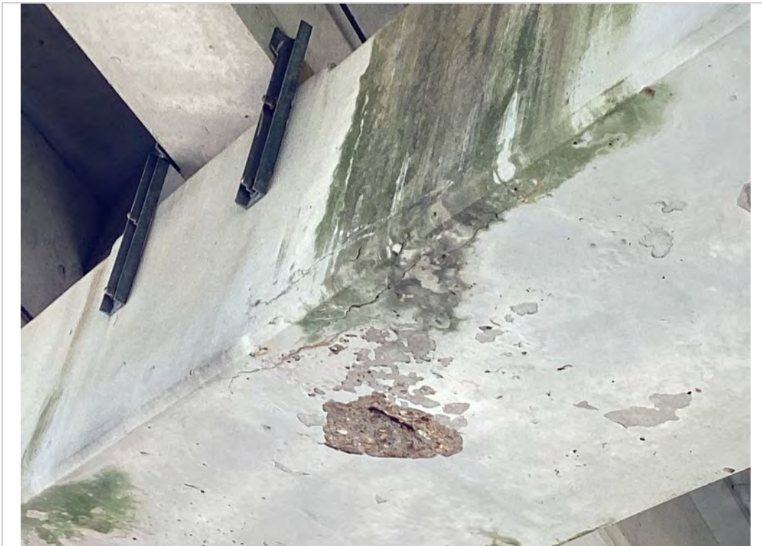
Bent 2 impending spall
