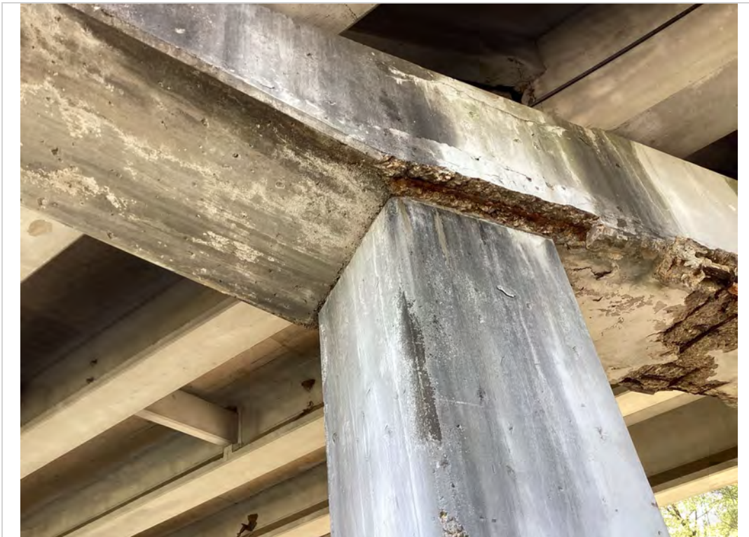
Bent 1 Cap spalled to steel on rear side over pile B
