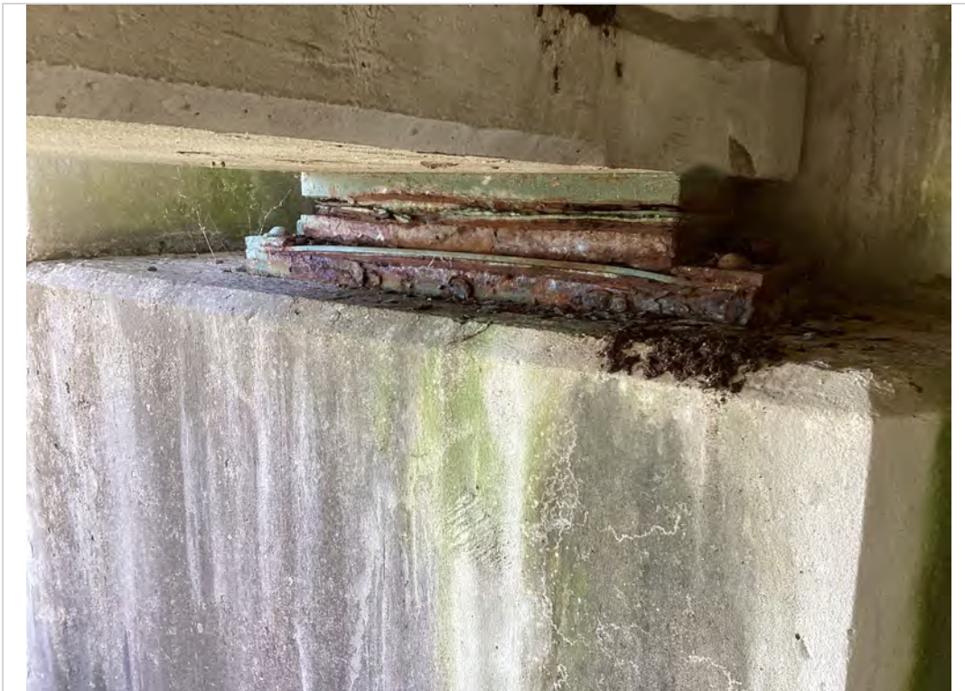
Abutment 1 bearing E. Heavy Corrosion
