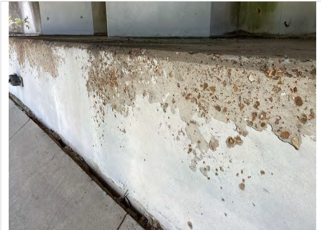
Abutment # 2 cap, scaling
