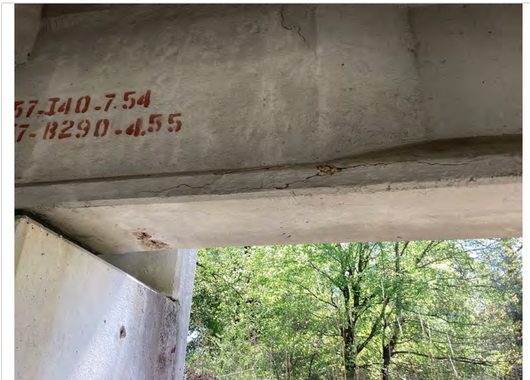
Span 1 concrete I-beam "A" impending spall and spall to steel
