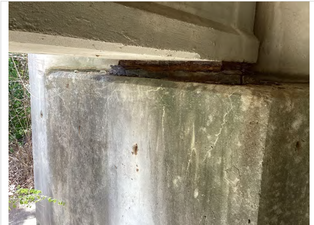
Abutment # 2 poor bearing under beam A
