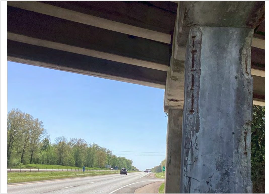
Bent 3 Column B spalled to steel on Right side Direction of Route
