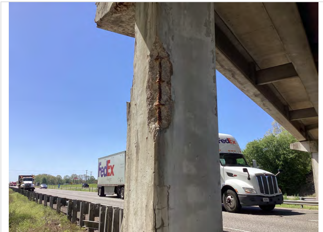
Bent 1 column A Right side. Beginning to Spall and spalled to steel
