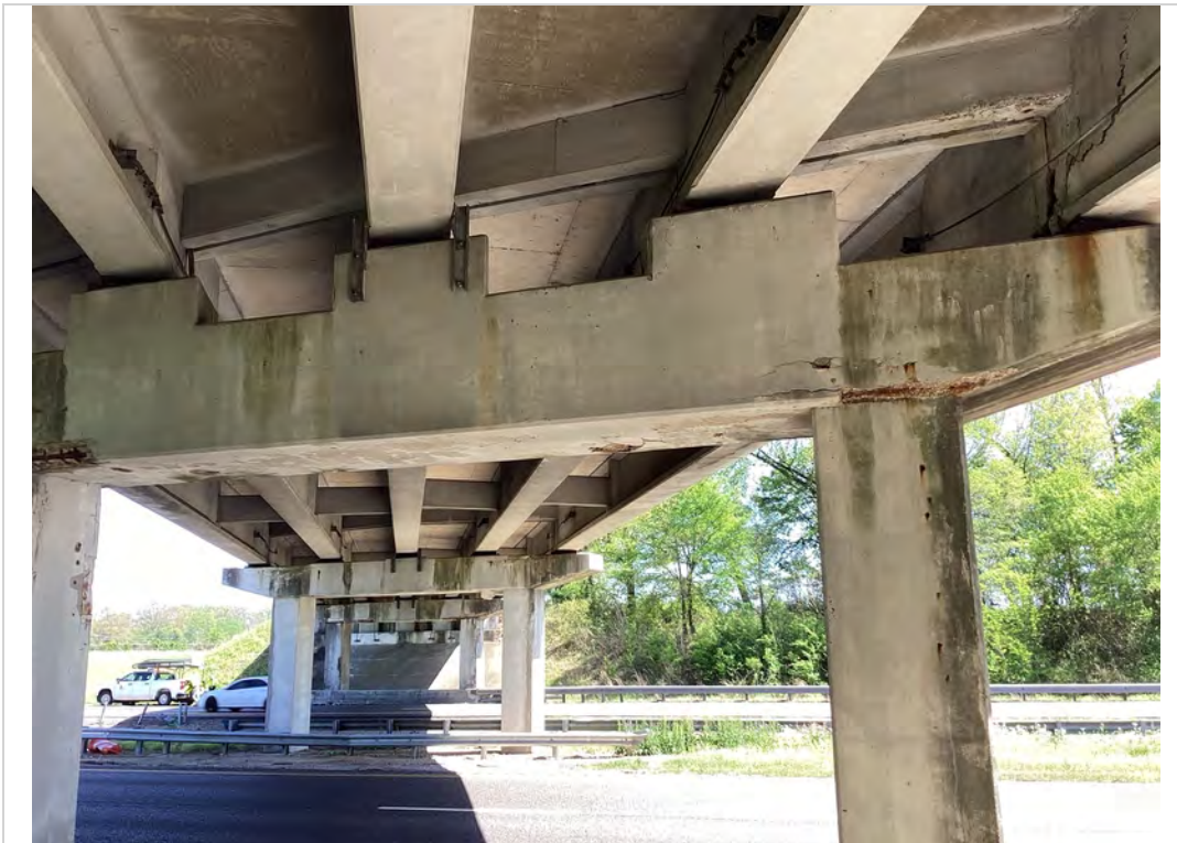
Bent 3 rear spall to steel and impending spall
