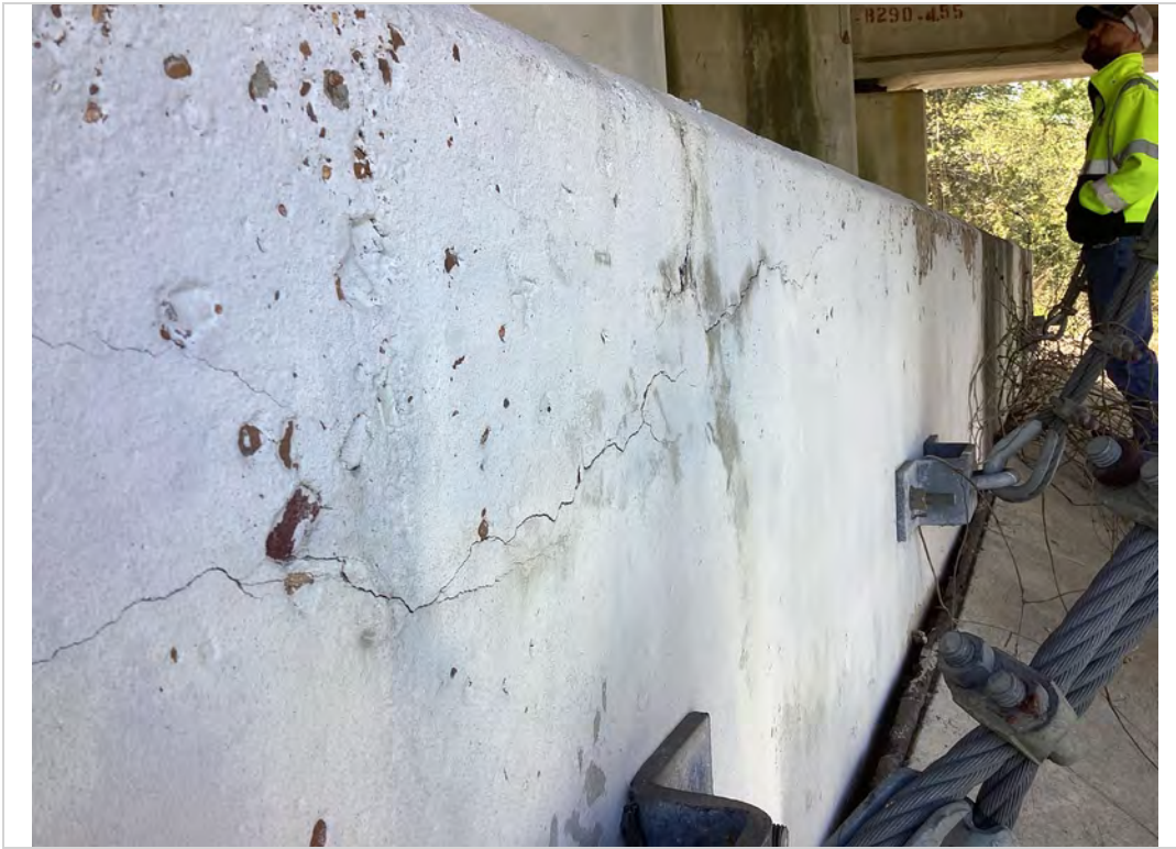
Abutment 1 cap fine cracks up to 1/16"
