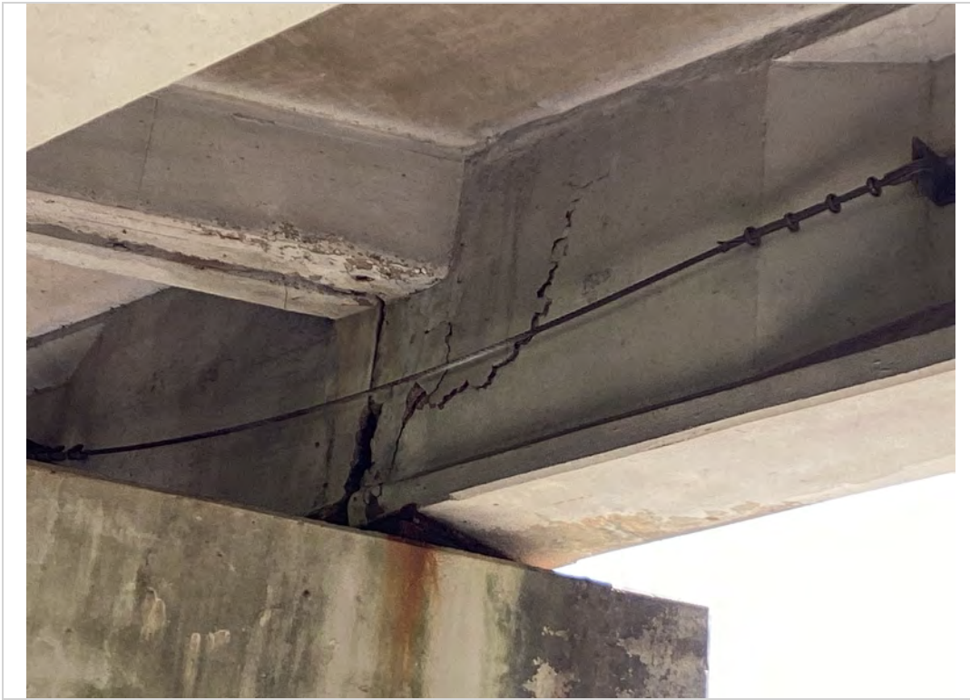
Spall steel beam a span 4
